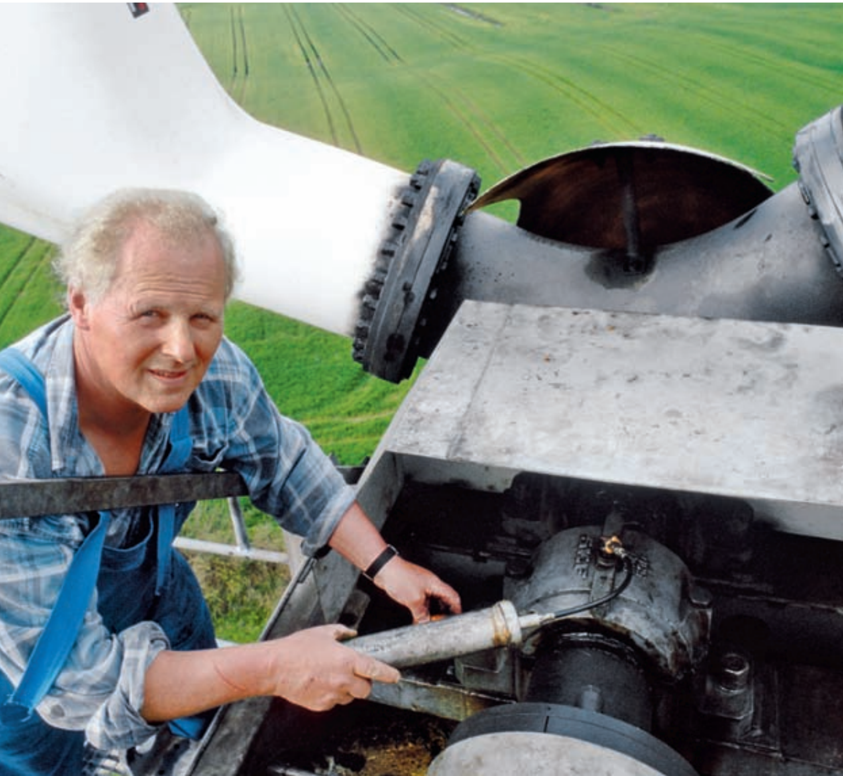
Do-it-yourself: Claus Engelbrechtsen of Breklingfeld, Germany, maintains his Nordtank himself. It continues to run perfectly. He installed the 65-kilowatt turbine in 1987; it was the first Nordtank in Germany. He bought it second-hand in Denmark in 1985 and connected it to the grid after months of type-testing in Schleswig-Holstein.
